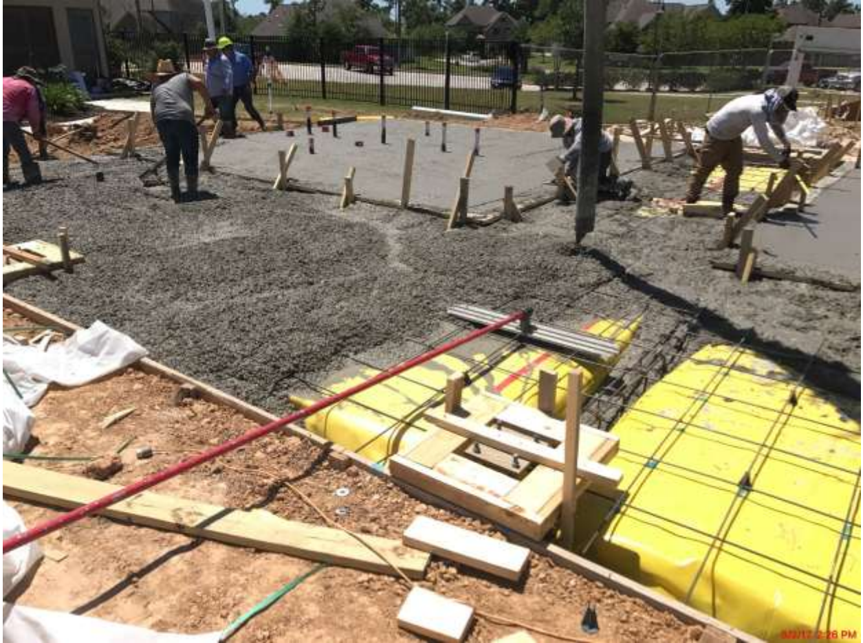
Description: Poured the concrete piers, rough graded the subgrade, installed the under-slab plumbing, in the process of relocating the electrical feed to the existing lights.
